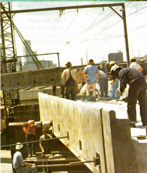
Top: Tracks and old bridgework removed, the piers and abutments are prepared to receive the new beams.
