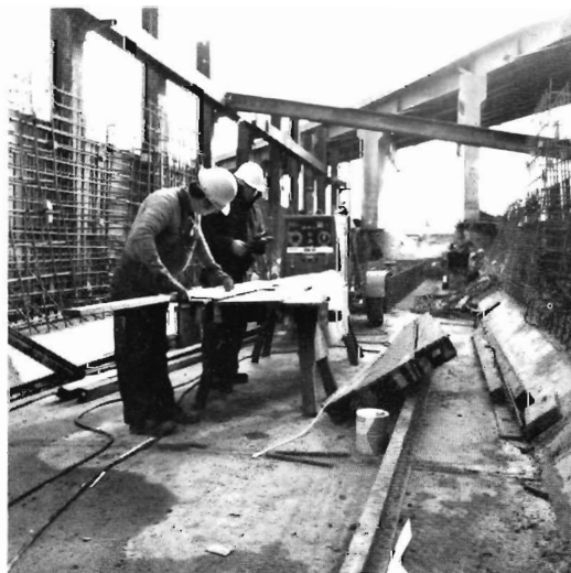
Left: Station foundations at Parliament in Spring Street. Above: Workmen on the job at North
