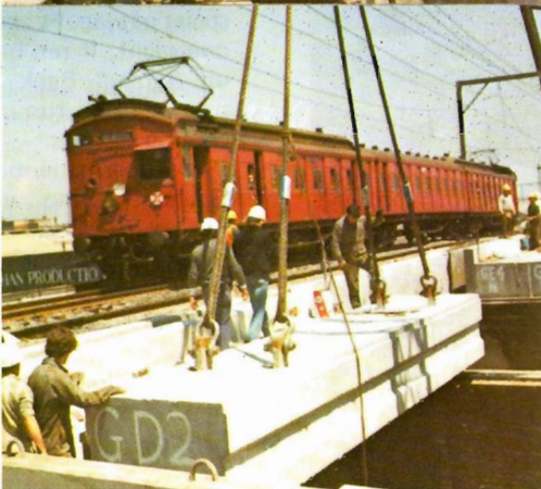
Bottom Left: A Tait train crosses the completed section of the bridge while work nears completion on the second section.
