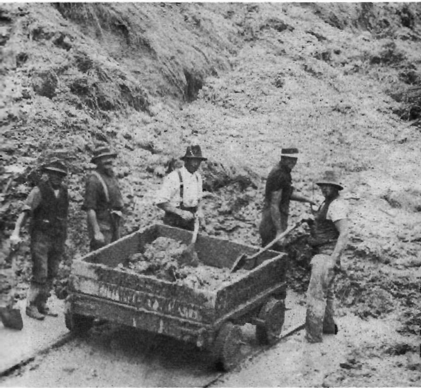
Heavy rain in South Gippsland during November in 1934 also caused a landslide onto track at Kardella. And the job of clearing the line back to depression days was by shovel, elbow-grease and trolley.
