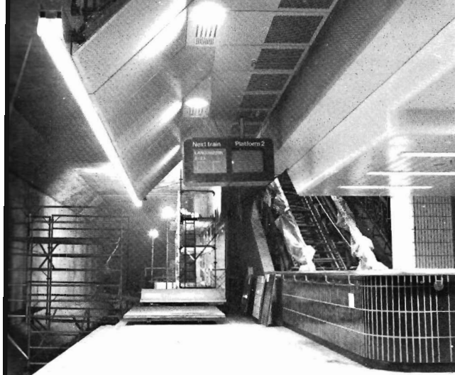
Museum station takes shape in readiness for its opening towards the end of next year. The escalators were installed last month.
